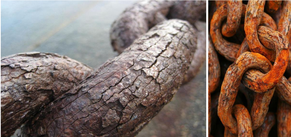
Il. 13. The chains from the Golden Gate bridge near San Francisco, source: pinterest.com [12.03.2018]
